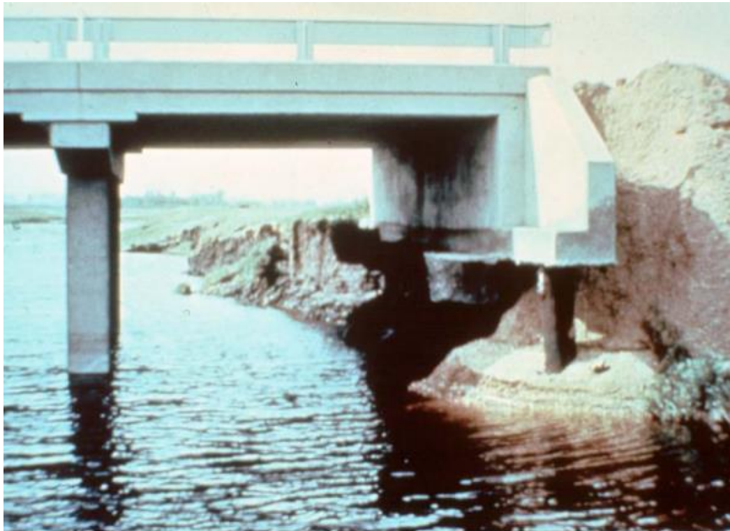
Figure 13: Bridge Abutment Scour
