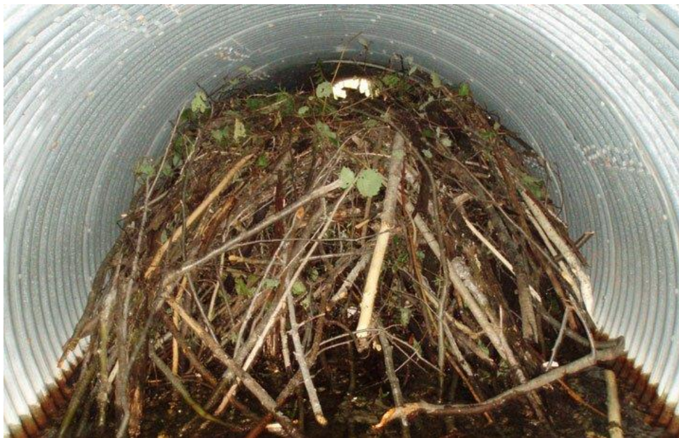
Figure 12: Caltrans District 10 Clogged Culvert
