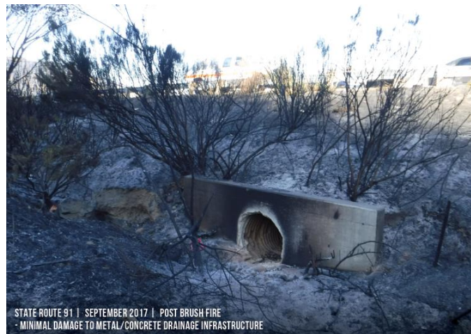
Figure 21: Metal Pipe and Concrete Headwall Post-Fire
